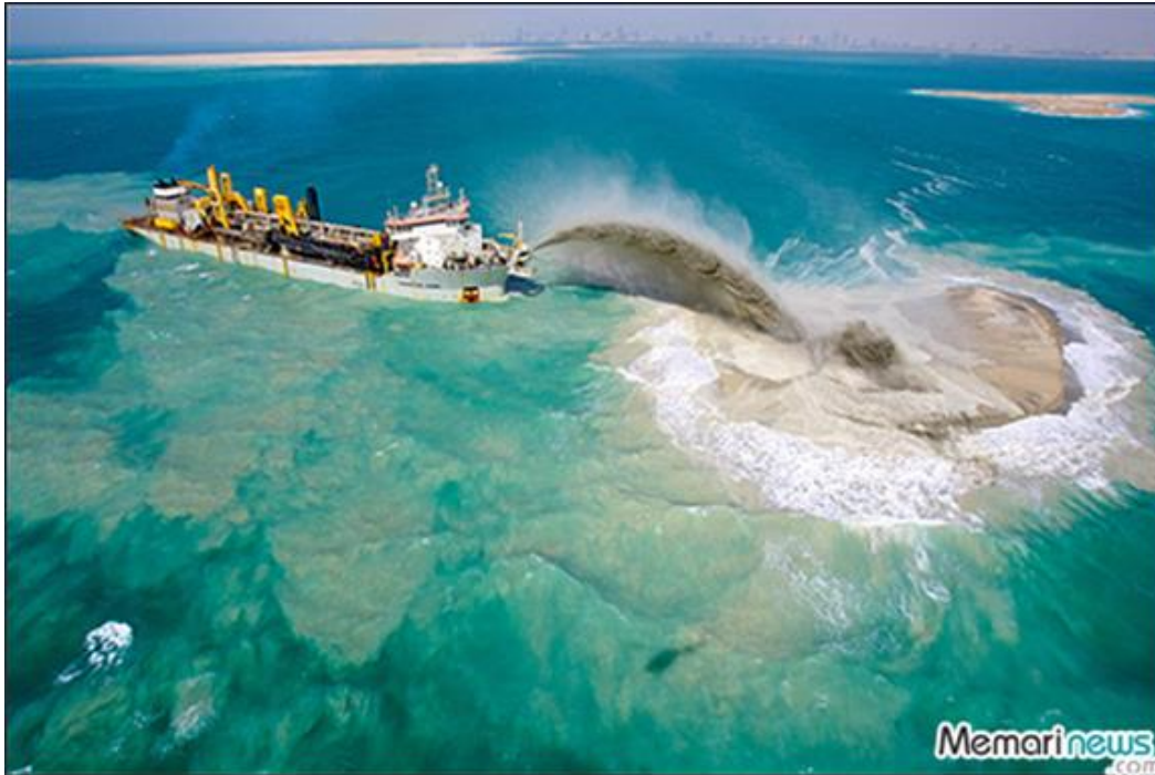
Figure 1. Adding the huge amount of sands and soils into the sea for building artificial island.
